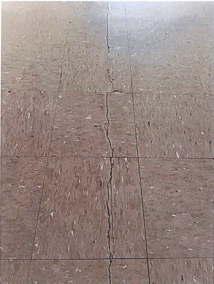
Hall Cracking Areas
